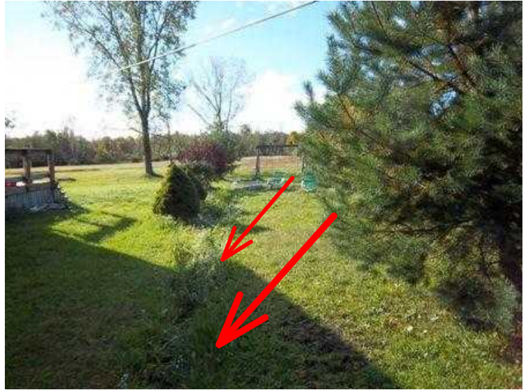
#6 Ditch at easement line. Ditch was made when Mr. Melms built his house. The engineering company obviously graded the lot to the easement line. Easement is in plot plan.
